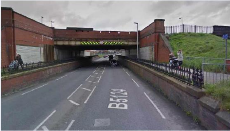
Essential work at Devonshire Road Bridge will start on Monday 4 June, 5am as Blackpool's major bridges improvement programme moves into its final stages.
